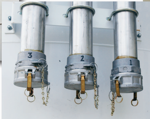
Numbered loading connections
