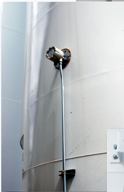
Monitor level sensor
